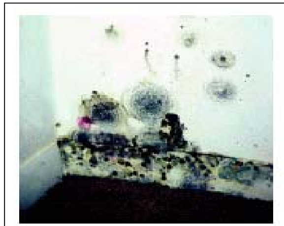
Figure 1: Mold growing in closet as a result of condensation from room air.
